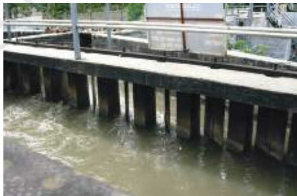
Fig. 13.4 Grit and sand removal tank
